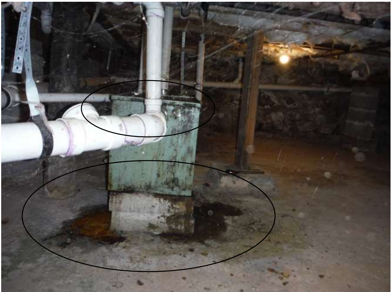
Figure 20 Grease on floor and the trap in crawl; have evaluated for clean-up, check grease trap for level and leaks.
