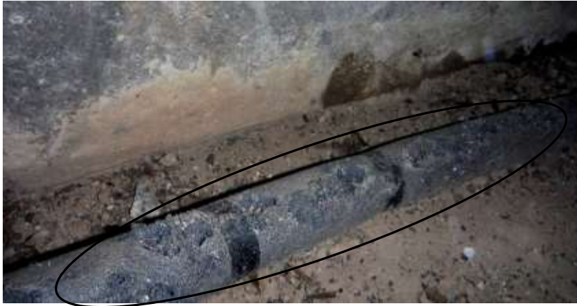
Figure 19 Chewed pipe insulation in crawl space; have rodents/mice addressed by a licensed Pest company. Recommend a structural mason repair/seal/repoint foundation.
