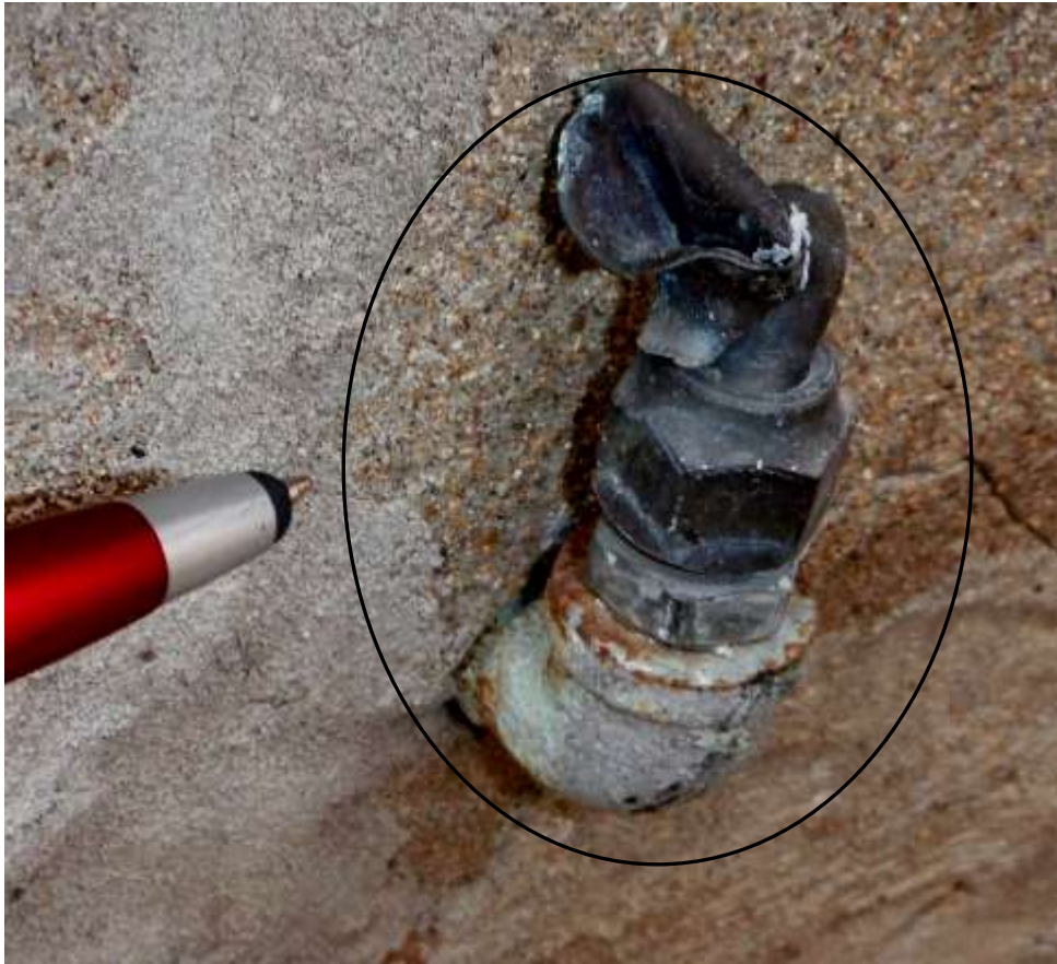
Figure 9 Further evaluate abandoned piping on exterior left side in rear by a licensed plumber. All abandoned piping should be removed and foundation sealed. Rule out any buried oil tanks on property.
