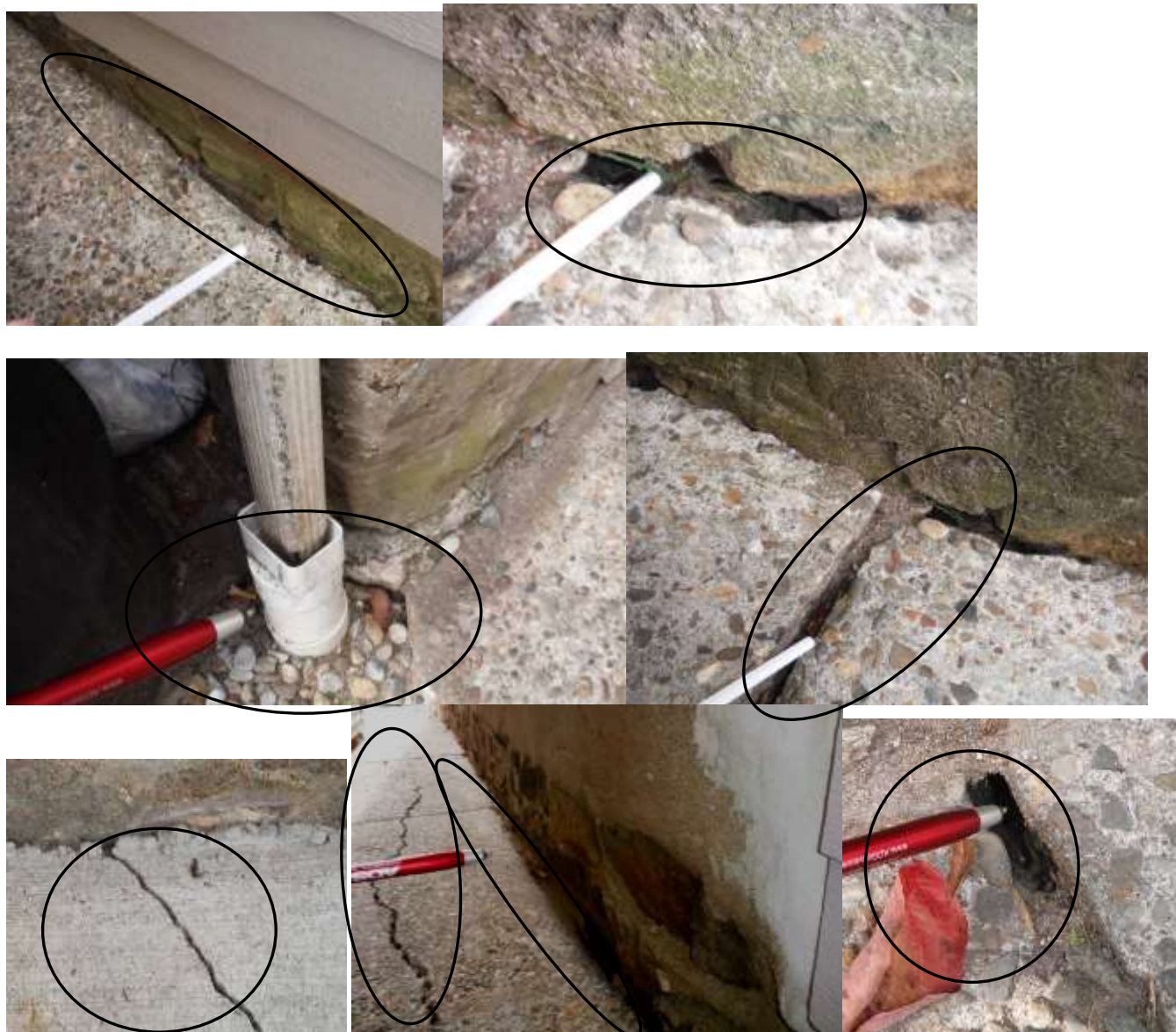
Figure 1 Examples of gaps, concrete cracks or openings at the sidewalk/foundation junctures; have a contractor make repairs along with proper drainage. Left side of building had poor drainage; right and rear right sides were inaccessible.
