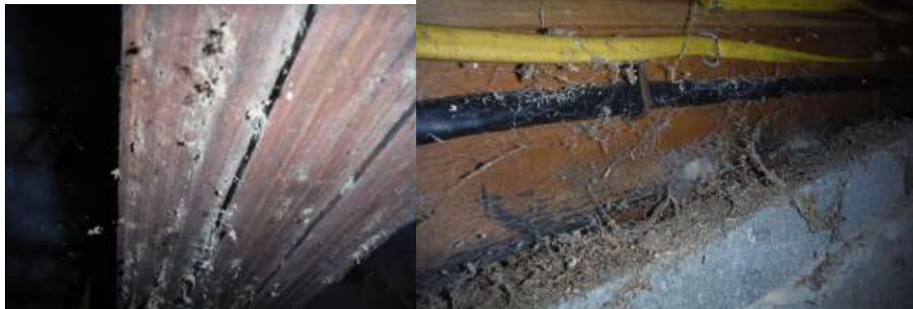
Figure 16 Example of carpenter ant frass & bodies; on insulation (ceiling & pipe), floor, joists, foundation, etc. Conditions in crawl are wet/seepage/high humidity; have all conditions on exterior and crawl corrected ( ventilation, humidity, seepage, etc.).
