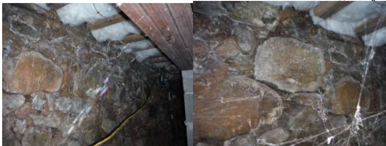
Figure 11 Example of efflorescence ( white salts), seepage, wet/water stains, moist humid conditions in the crawl space.
