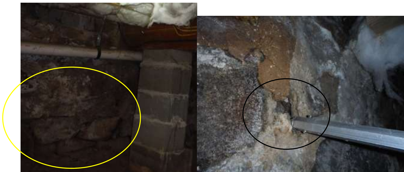
Figure 17 Example of holes, gaps, missing mortar on stone foundation. Recommend a structural mason evaluate foundation and make repairs. Recommend a structural engineer (PE) evaluate bulged wall(s) on left. The right side and rear of exterior was inaccessible.
