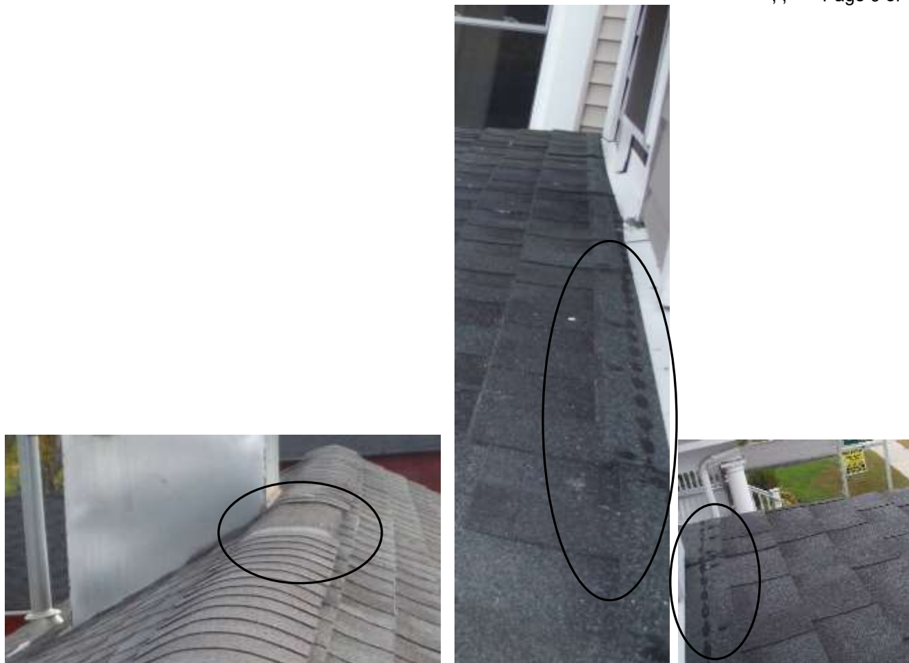
Figure 2 Appears to be missing ridge cap shingles near roof vent. Tarred nail heads; tar will crack /potential leak points.
