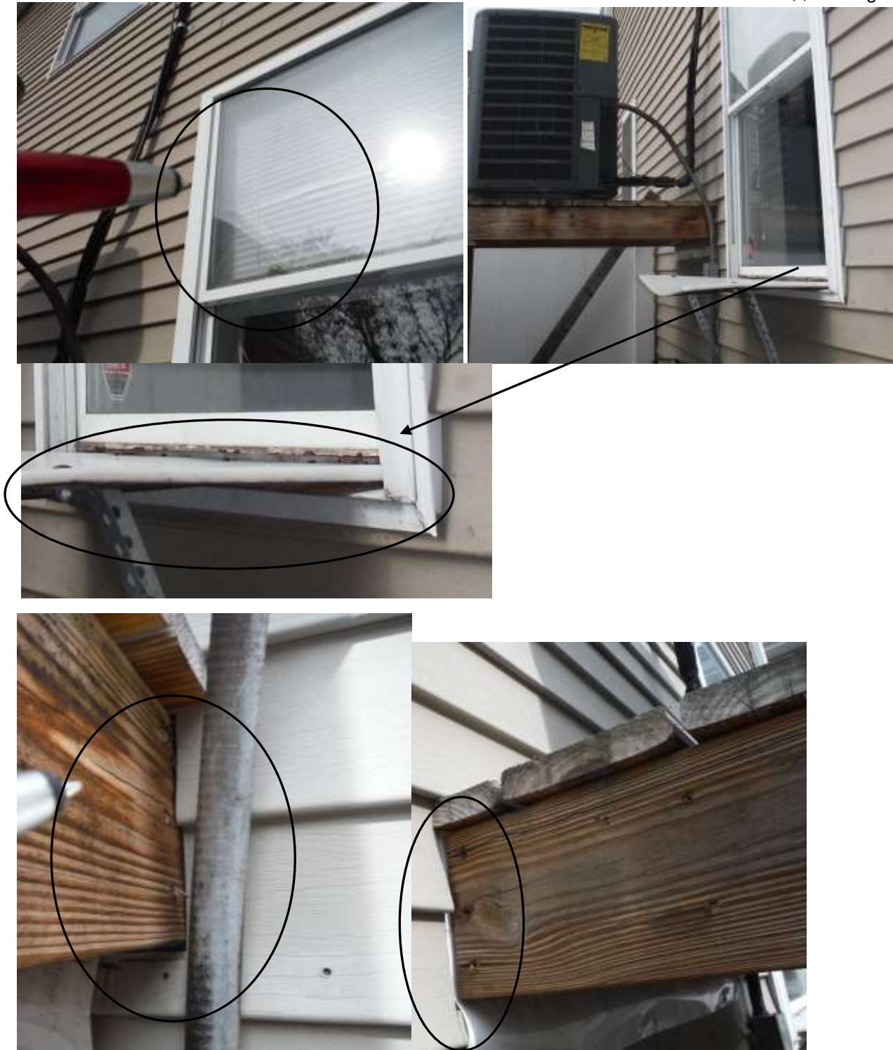
Figure 10 Cracked window pane, bent frame and not flashed properly; rear kitchen area. A shelf was added to this window; appears to be for a window A/C unit. There was improper flashing around the wood shelf for the Goodman condenser; water entry points.
