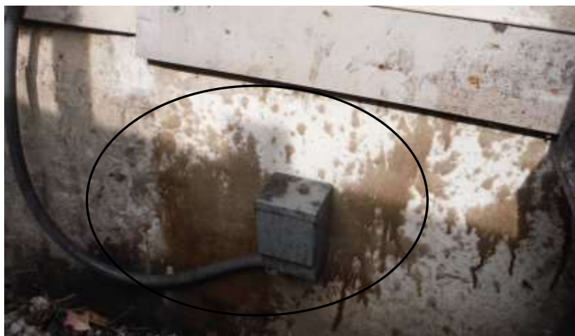
Figure 8 Recommend protecting the A/C disconnect from grease/garbage; can damage electrical cable and box.
